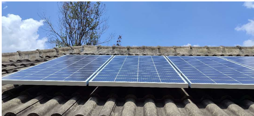
Gambar 4. Panel Surya Terpasang
